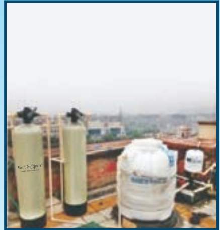
Sand Filter & Softener Plant
