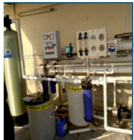
2000 LPH RO Plant
