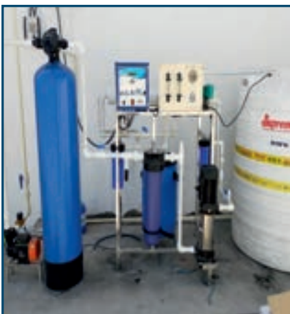
250 LPH RO Plant
